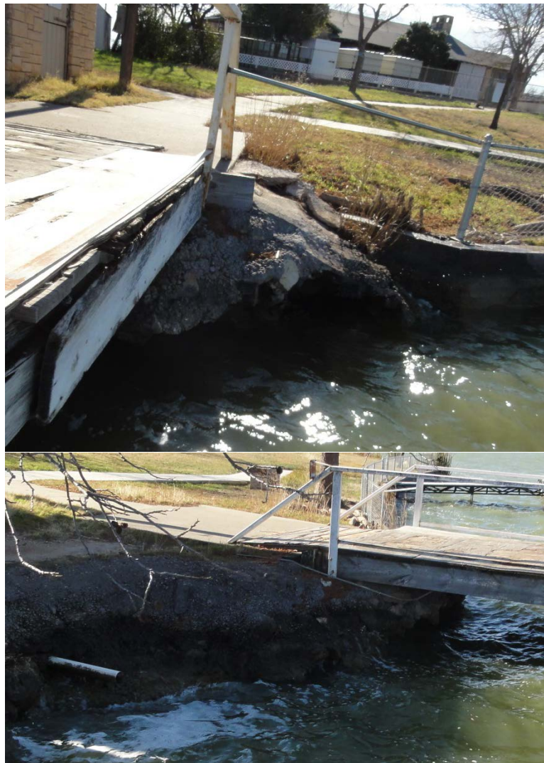
Figure 7: Undermining at Abutment
