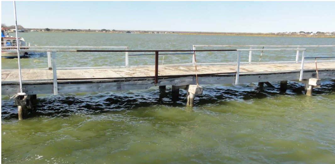
Figure 6: Distressed Floor Framing
