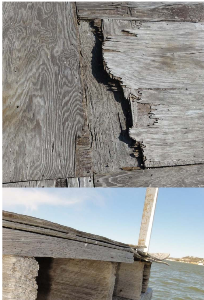
Figure 8: Damaged Walking Surface
