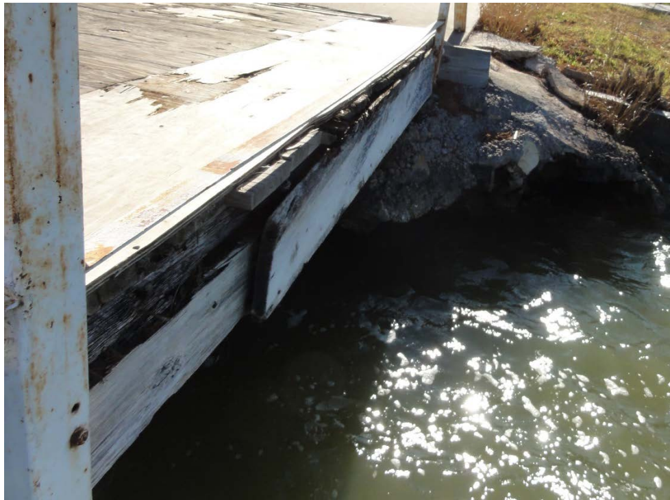
Figure 5: Distressed Floor Framing
