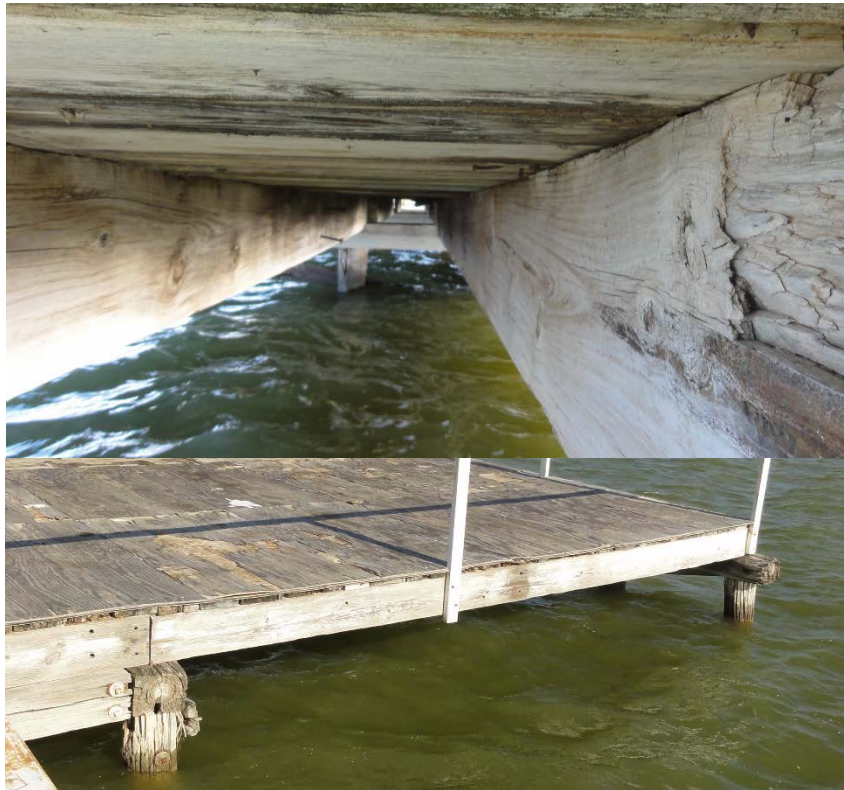
Figure 4: Typical Sagging Floor Framing
