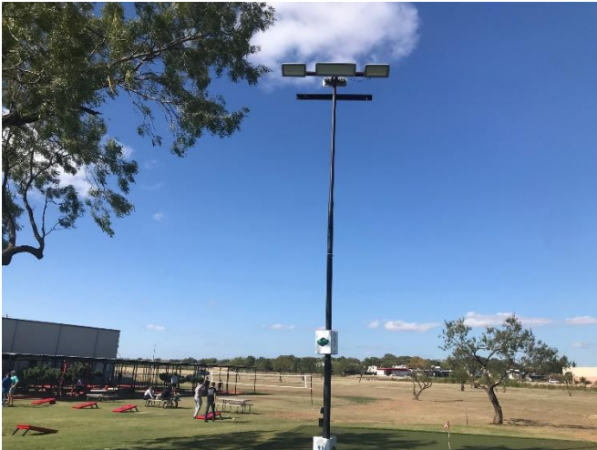
EXISTING LIGHT FIXTURE
