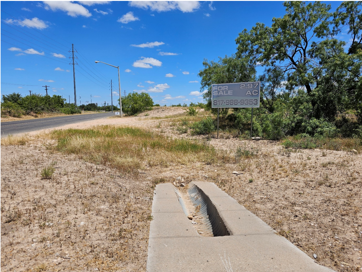
Entrance off of The Crossings site where the Attorney General's Building is located. It shows the existing drainage structure carrying water from across The Crossings state property to this site where it naturally flowed.
